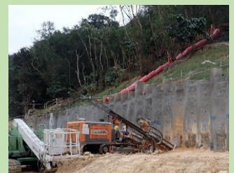
安裝挖掘與側向支撐系統上的 的錨杆 Installation of Tieback of Excavation and Lateral Support System
